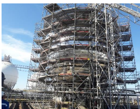
Insulation of the ball hopper
