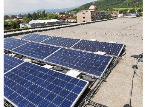
Weighted structure of a PV plant, using concrete elements
