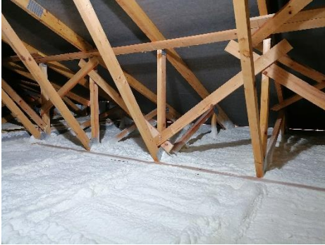
Spraying from above (from the attic space) into the truss structures on OSB board
